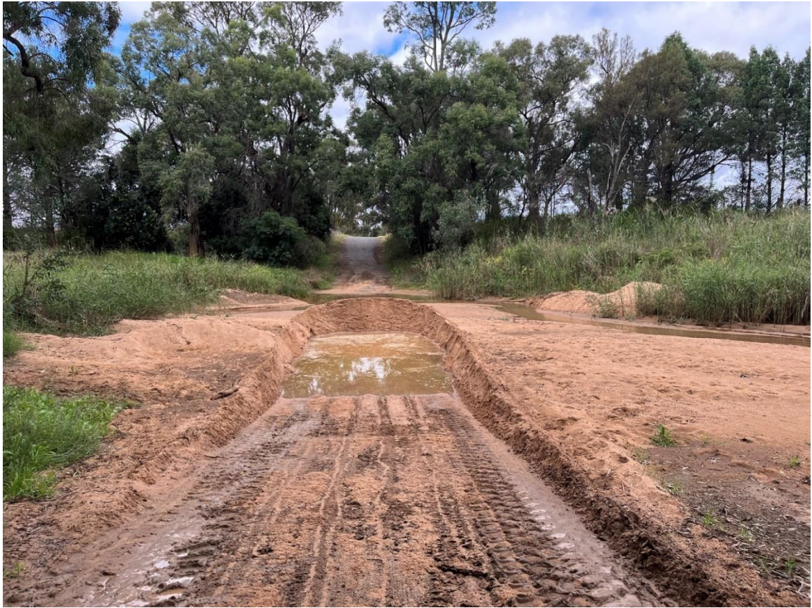
Photo 3 – Merrygoen Creek Causeway on Yarrow Road, Mendooran – Council clearing all the sand from the causeway on the 20 & 21 April 2022
