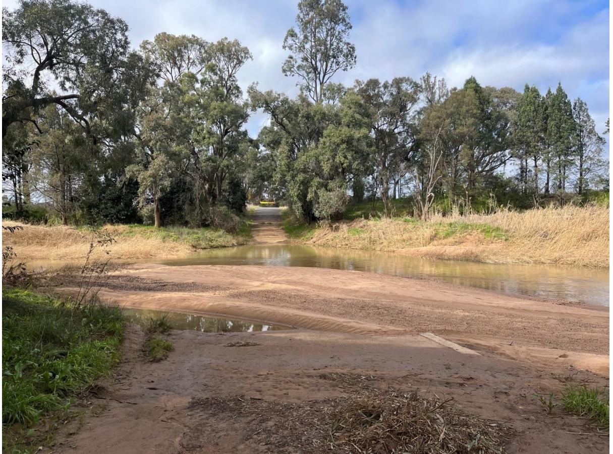
Photo 7 – Merrygoen Creek Causeway on Yarrow Road, Mendooran – 25 August 2022
